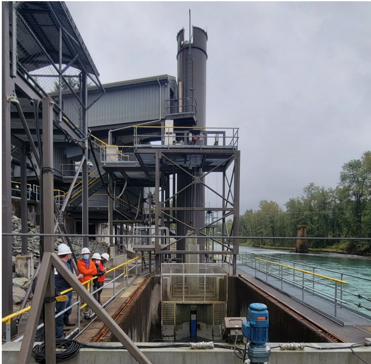
Figure 8. Fish Lock at the Trap and Transport Facility on Baker River Operated by Puget Sound Energy
