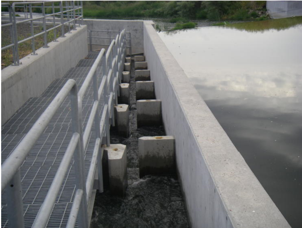
Figure 6. Crooked River Central Vertical Slot Fishway near Prineville, Oregon
