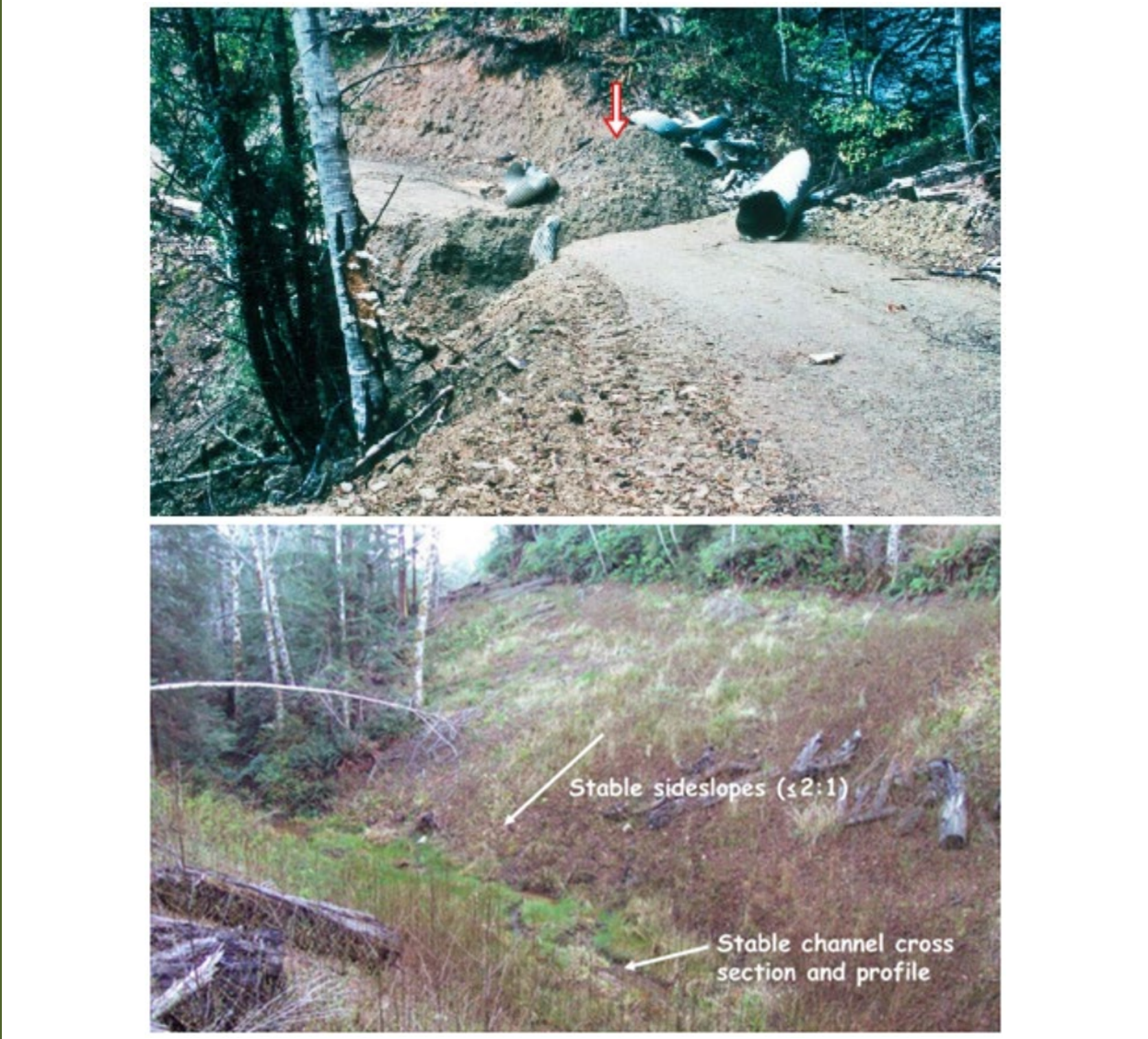
Figure 6 Top Panel: Poorly “Decommissioned” Stream Crossing with Excavated Spoil Piled Next to the Trench (Arrow) That Could Easily Erode into the Stream. Lower Panel: Properly Decommissioned Stream Crossing, with 2:1 (Stable) Sideslopes, Adequate Channel Width for Flood Flows, a Uniform Channel Grade, and Sideslopes Treated with Erosion Control Measures (Figures 264 and 265 in Weaver et al. 2014).
