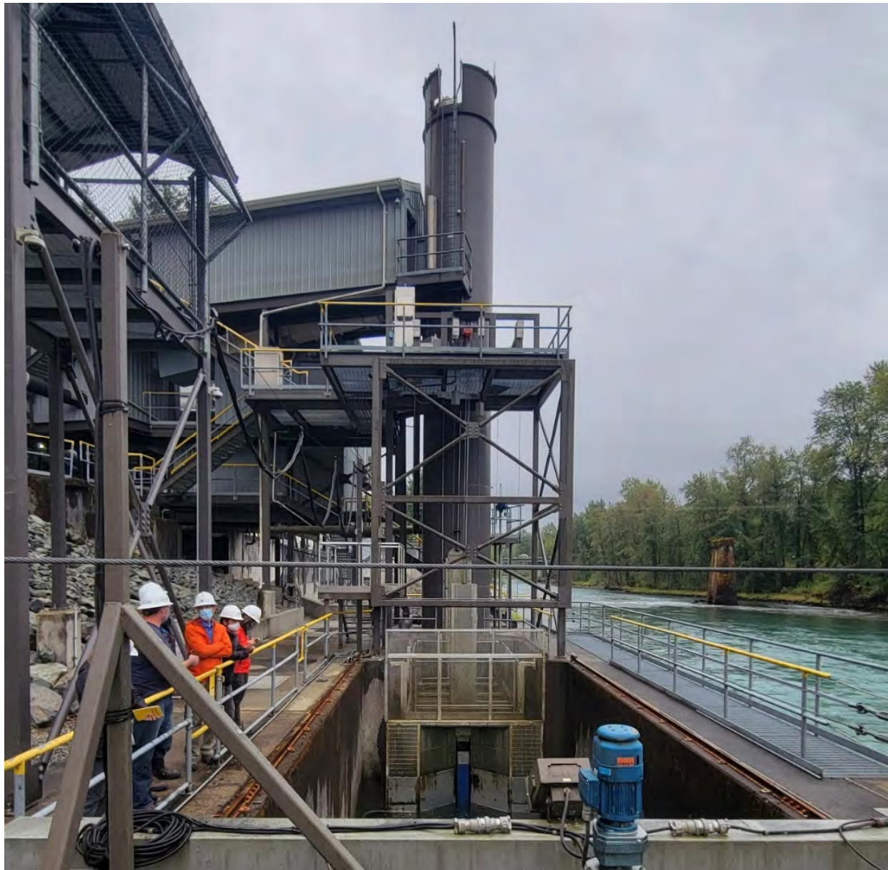
Figure 8. Fish Lock at the Trap and Transport Facility on Baker River Operated by Puget Sound Energy
